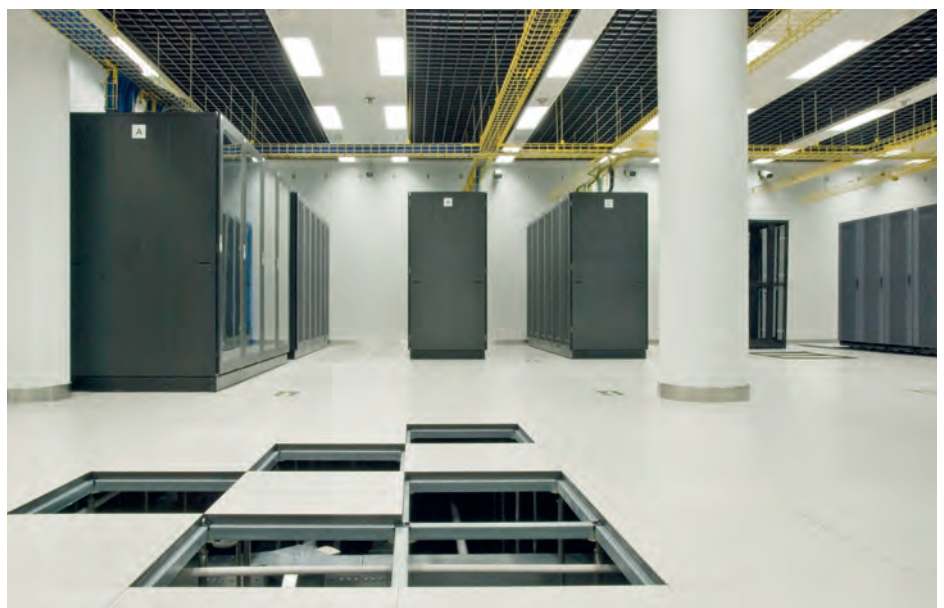
Siemens Beijing, Peking, China
